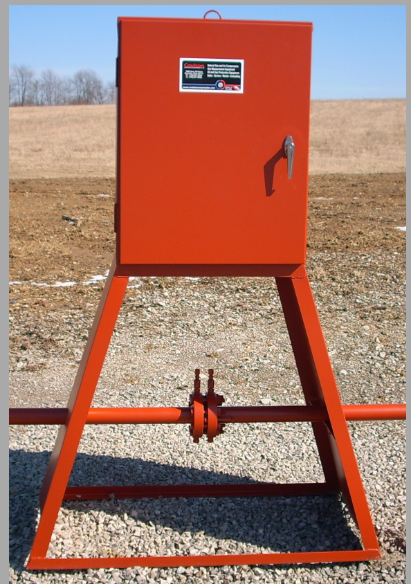
Standard Closed-leg Steel Meter Station
